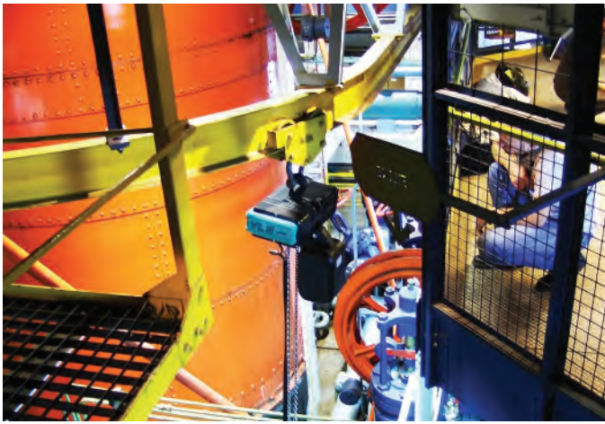
Fig. 6. Another view of the sub-basement equipment with a portion of the large orange accumulator on the left. Credit: France Languérand.
